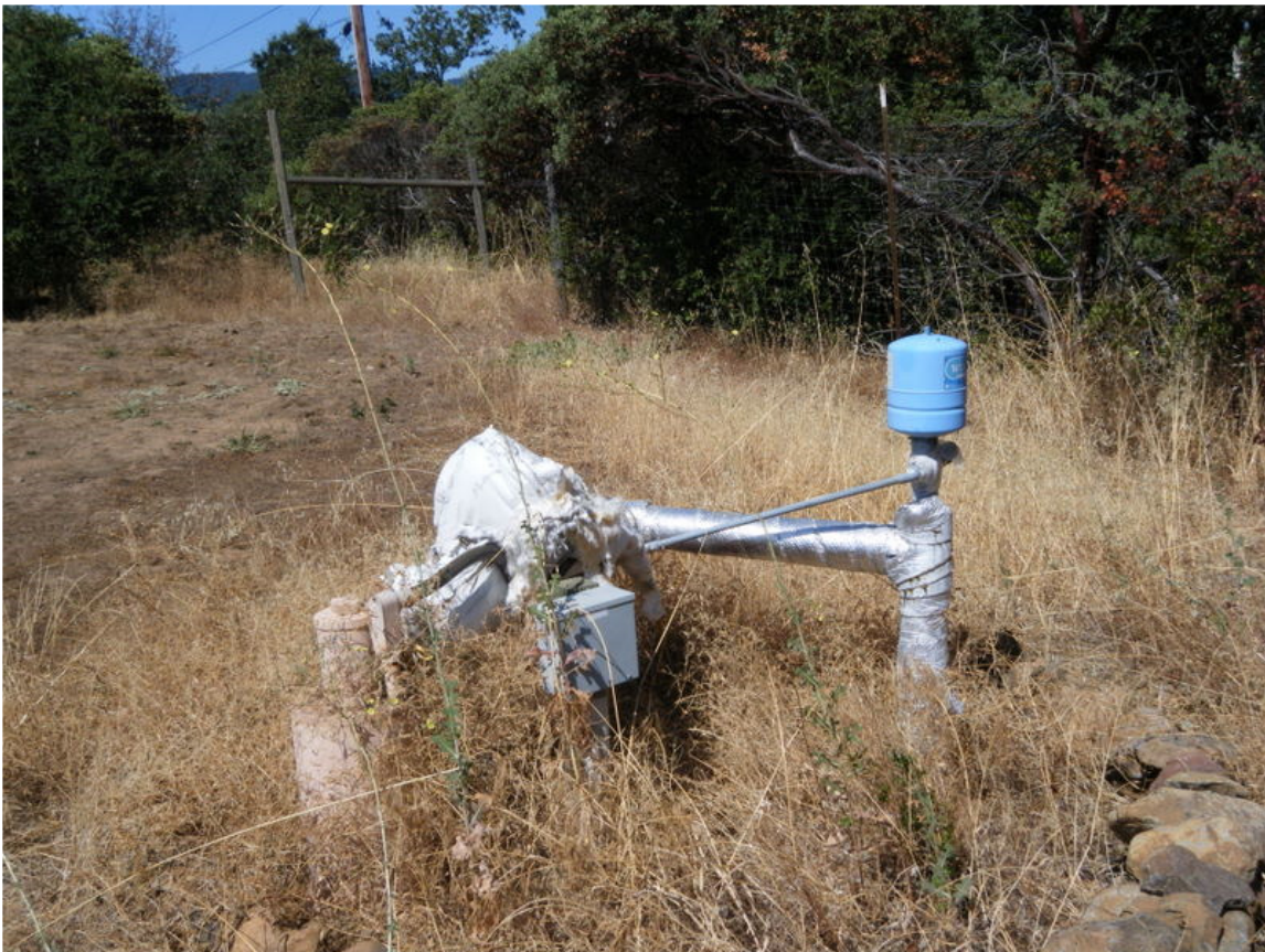
New (2001) well with 8" casing.
